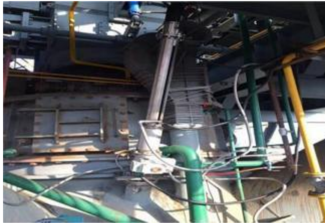
picture 1 HIRDA - BF Blast furnace charge surface infrared thermal imaging online temperature detection and analysis system product and installation diagram
